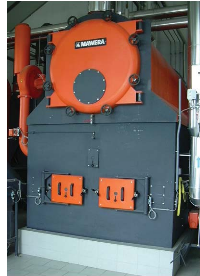
Caldera de biomasa para district heating (850 kW)
